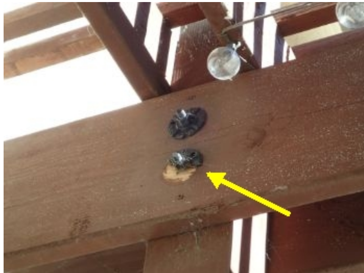
One of the lag bolt collars is cracked, and missing. Recommend repair.
