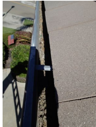
Clean gutters: Significant amounts of debris evident.
