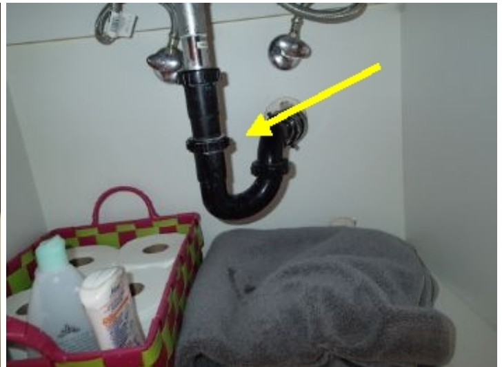
Drain line leaks under sink. Upstairs left sink. Needs to be repaired.
