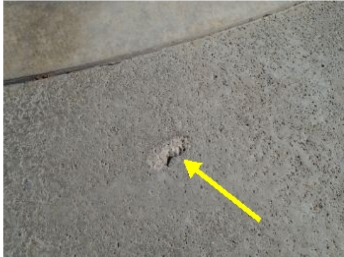
Driveway in good shape for age and wear. One area where a chunk of concrete is missing.
