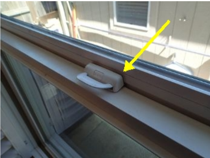
The window in the master bath does not lock. Needs to be repaired.
