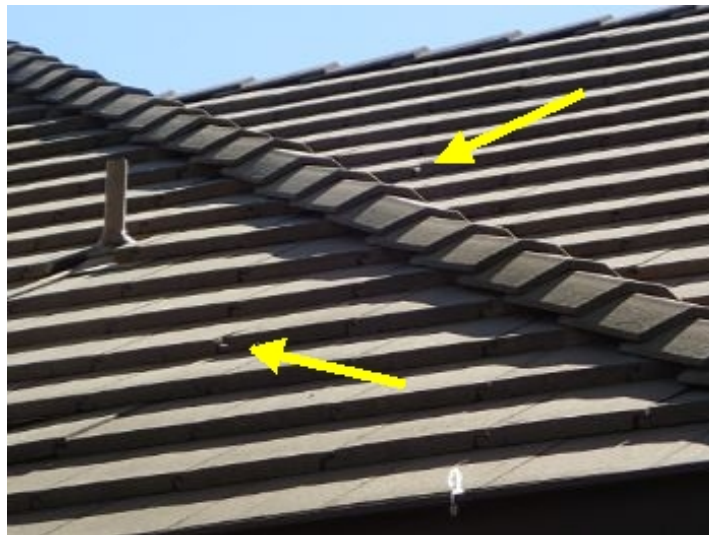
Several chipped tiles noted on the front of the house.
