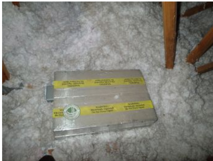
Whole house fan.
