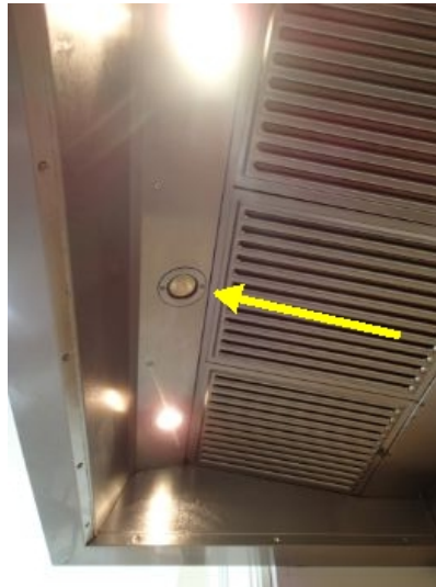
One light is burned out. Recommend replacing.
