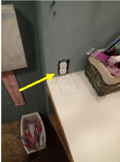
Outlet cover needs to be installed.
