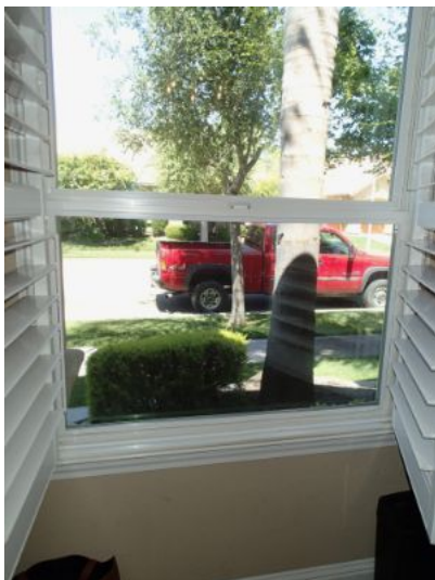
The office window is difficult to open, and close.
