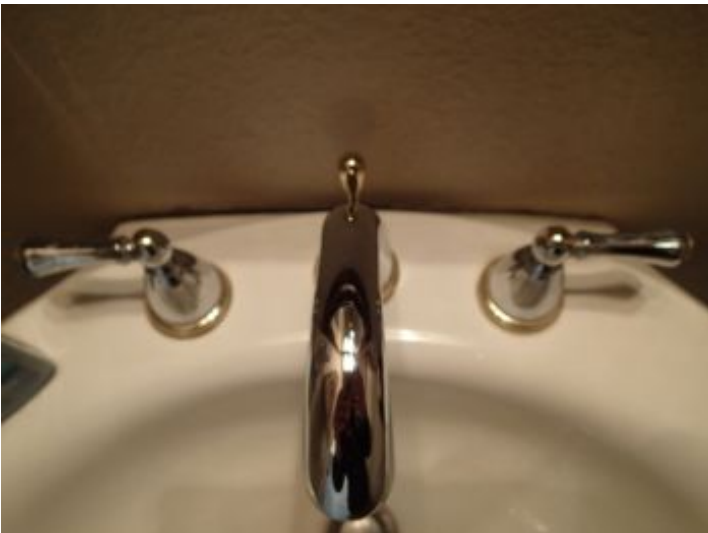
Half bath sink is loose. Recommend securing.
