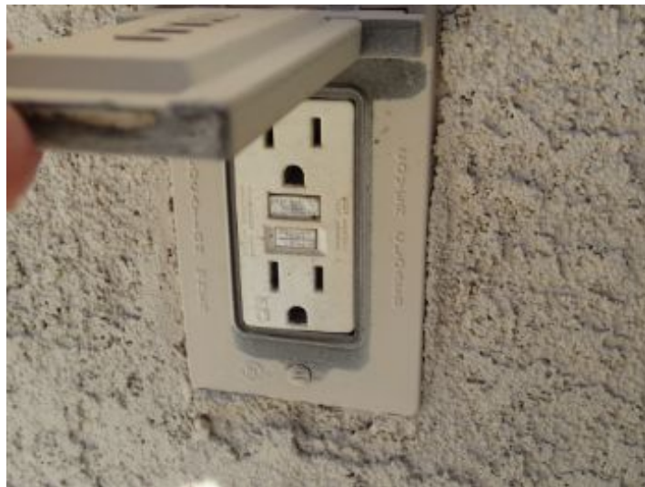
The rear patio GFCI did not trip when tested. Recommend repair or replace.
