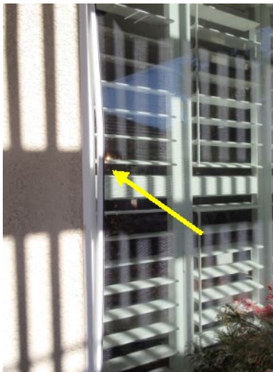
Damaged screen Dining room.
