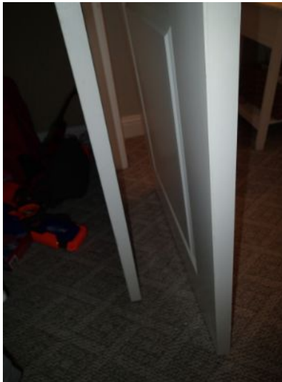
Closet door needs a bottom track guide.
