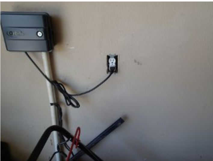
Missing outlet cover.
