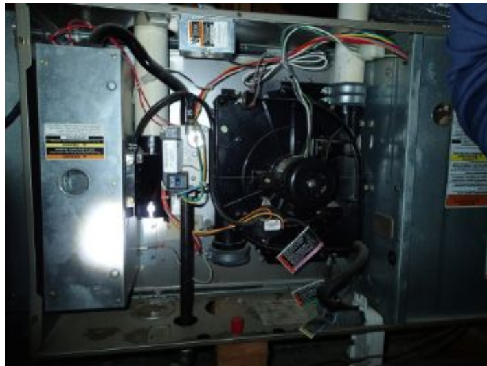
Furnace was operated, and found to function properly at the time of the inspection.
