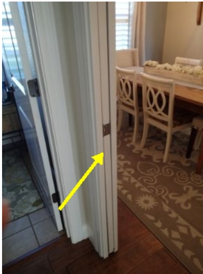
Dining room pocket door does not open or close properly.
