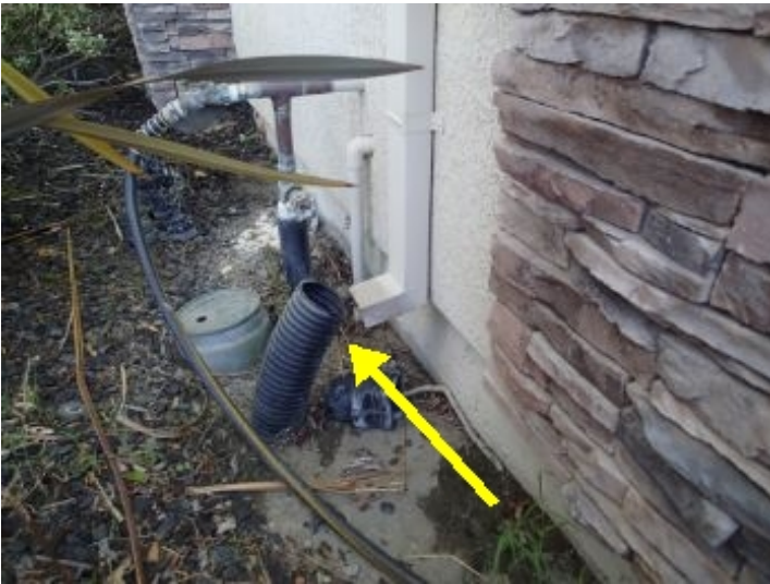
Downspout needs to be reconnected.
