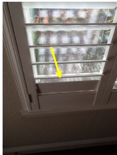
Dining area plantation shutter is damaged.
