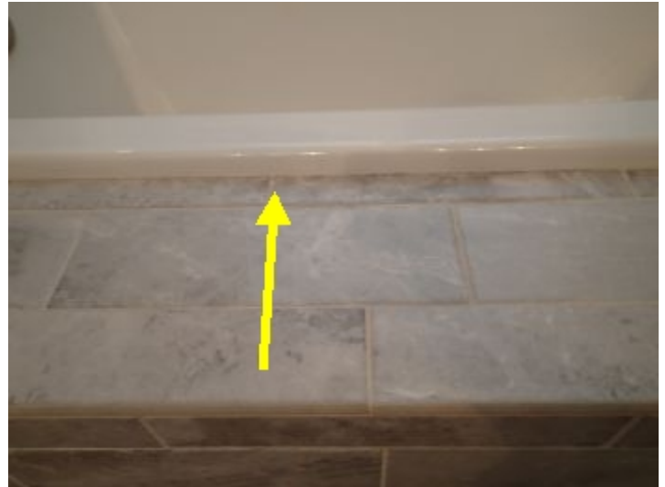
Recommend sealing around the master bath tub.
