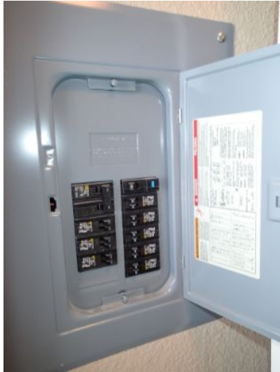
Sub panel in the laundry room.
