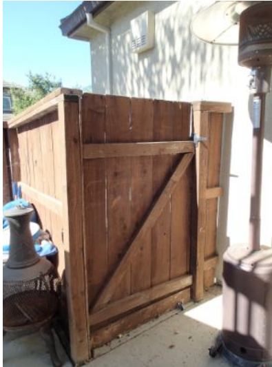
The gate is sagging and difficult to close.
