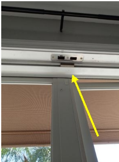
Hinged screen doors do not lock properly. Recommend repair.
