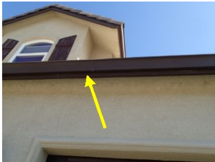
Gutters appear to leak at the seams. Recommend sealing.
