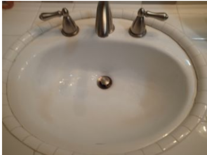
Stopper is missing/inoperable. Upstairs left sink.
