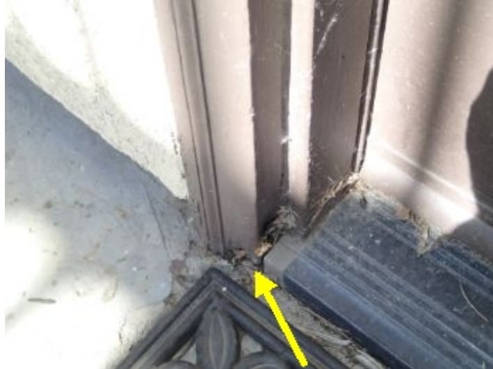
Garage door trim is rotted at the bottom.
