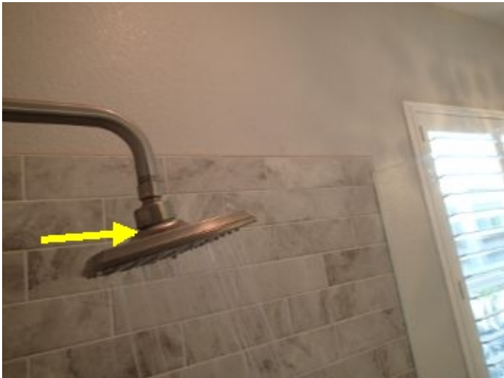
Shower head in the master shower has a slight leak when operating.
