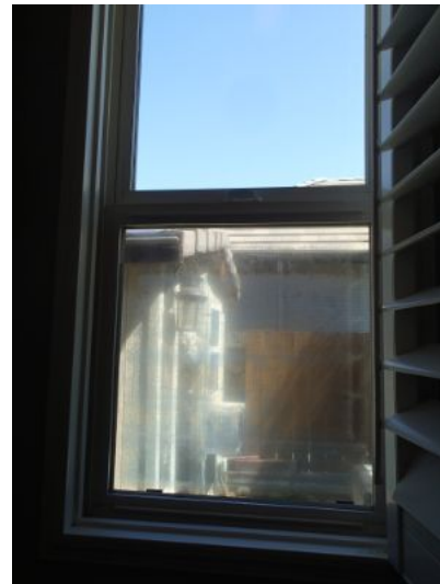
One or more window/s shows sign of loss of seal/condensation, recommend repair or replace to provide energy savings and prevent hazed window from limiting view out of window.
