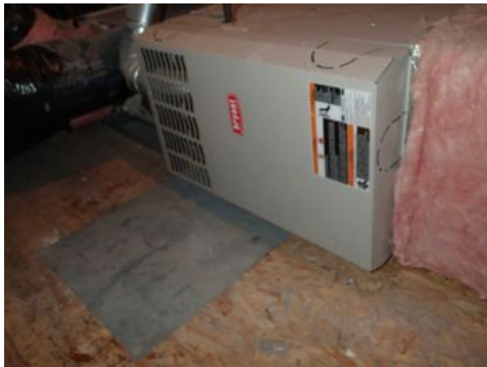
Relatively new high efficiency furnace in place.
