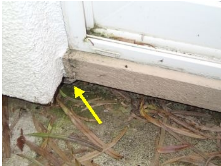
Wood rot noted under the sliding glass door. Recommend repair.
