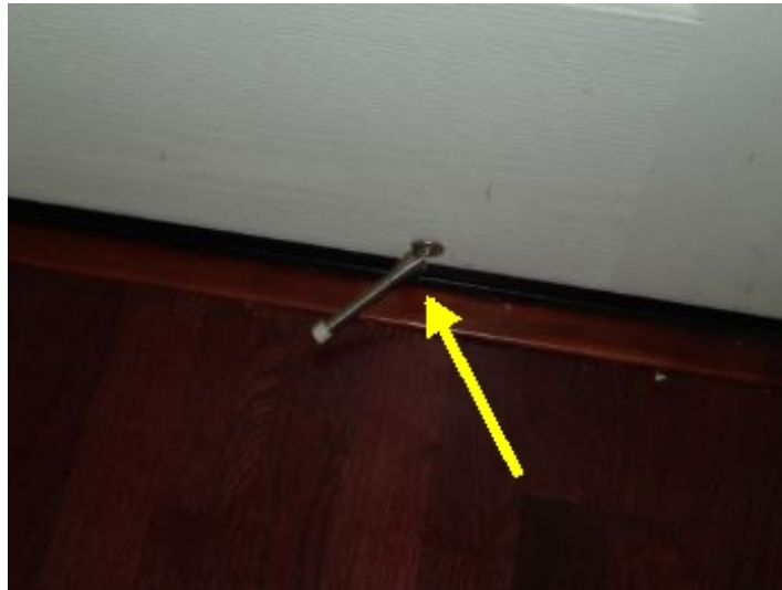
Stopper on the front door is broken. Recommend replacing.
