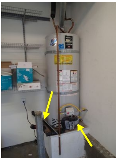
Rust noted at the bottom of the tank, and recirculation line.
