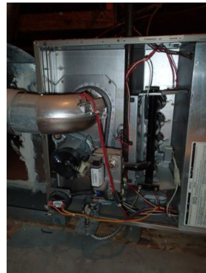
Due to the higher efficiency of this unit, this review is limited. Most areas are sealed and inaccessible. We suggest review by a licensed heating contractor if a more detailed review is desired.
