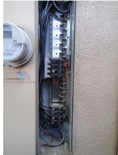
No major system safety or function concerns noted at time of inspection at main panel box.
