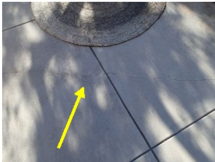
Common settlement cracks noted in the front patio area.
