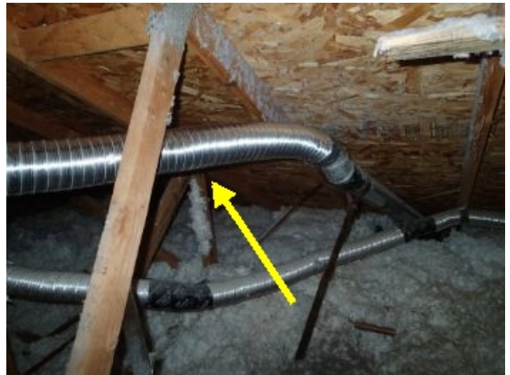
Dryer vent has been properly vented to the outside. 1/31/2019.
