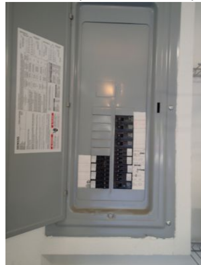
Subpanel in the garage. No hazards noted.
