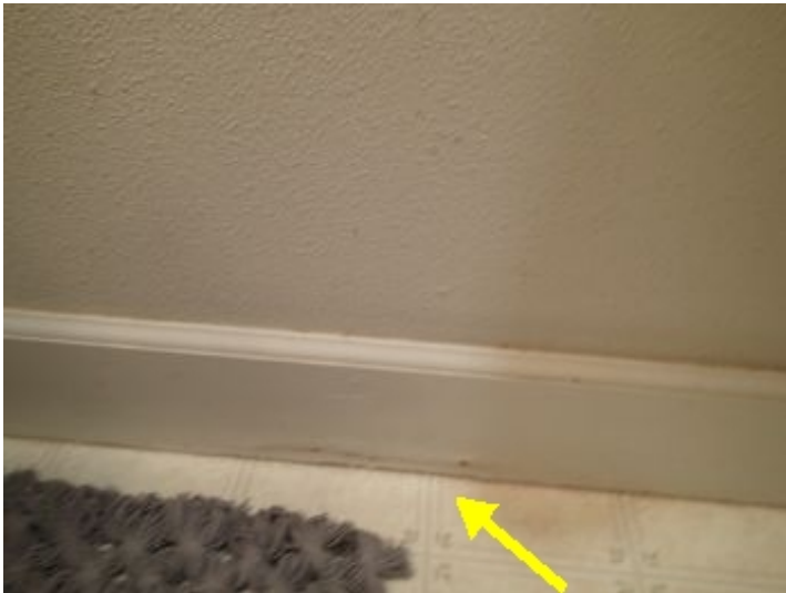
Slight water damage along the baseboard in the downstairs half bath.
