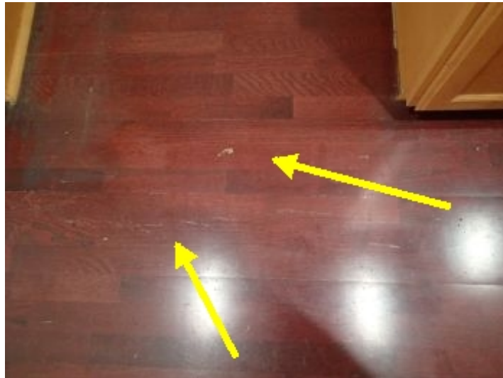
The flooring is scratched, and the finish is damaged in areas.
