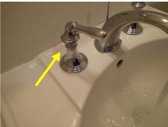
Faucet leaks at hot water handle. Downstairs half bath.
