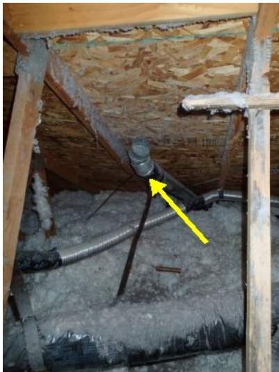
Dryer vent terminates in the attic. This is a fire hazard because it is releasing lint into the attic where the furnace is. The dryer vent also is releasing humidity into the attic which can cause damage to the structure. The dryer vent needs to vent to the exterior.
