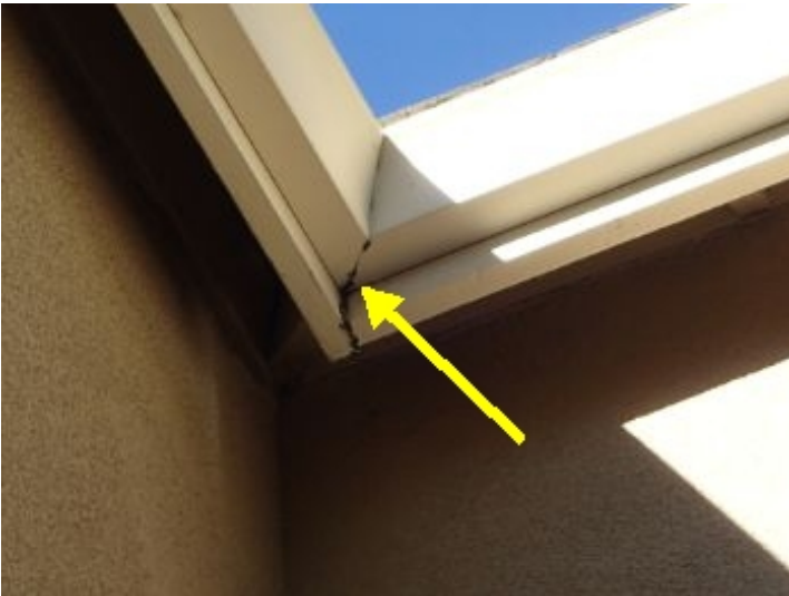
Gutter seam on the second story visible from the rear patio appears to leak. Recommend sealing.
