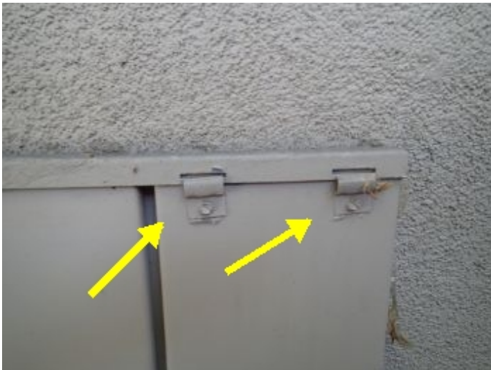
The main panel cover is loose. Needs to be secured.
