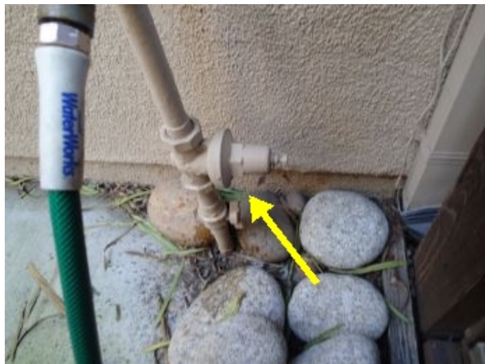
Pressure regulator noted. Needs to be adjusted.
