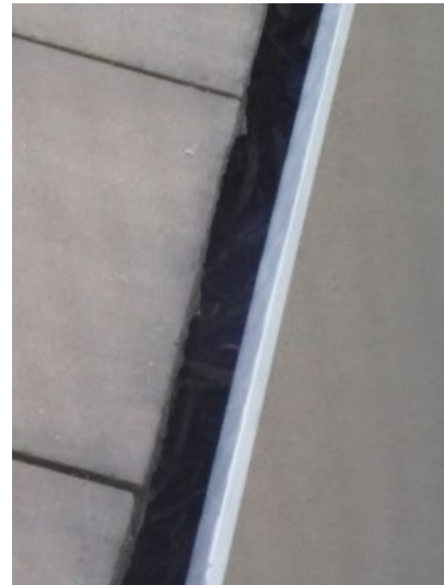
Clean gutters: Significant amounts of debris evident.
