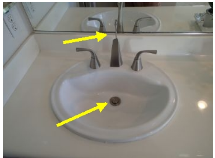
Stopper is missing/inoperable. Master bath left sink.
