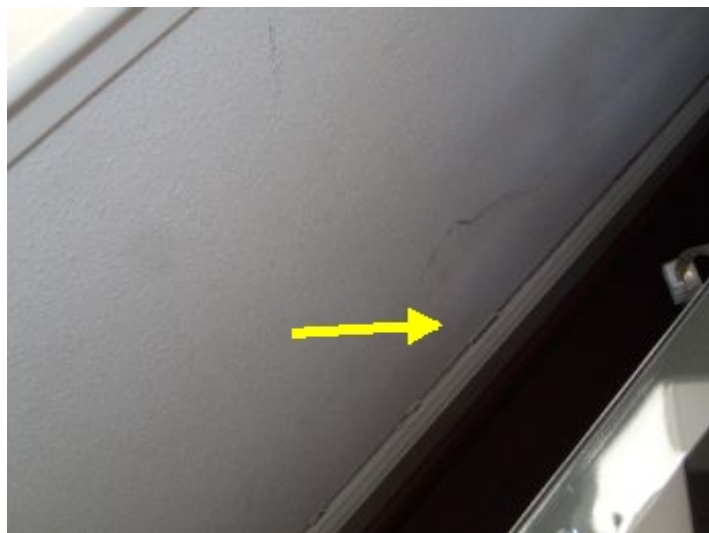
Baseboards along the living room north wall need to be recaulked.
