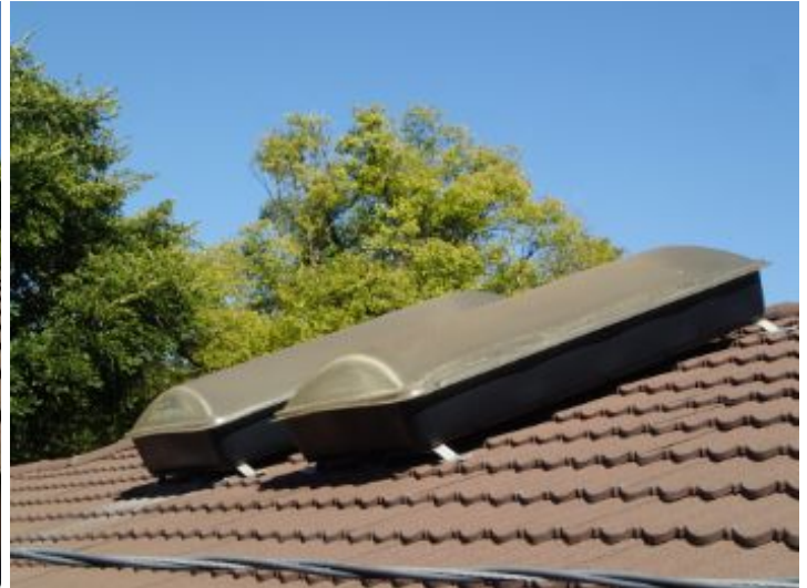
Old solar water heater panels on the roof. Recommend removing.
