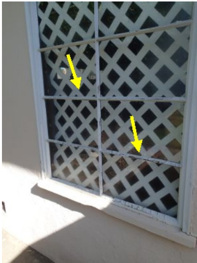
Garage window glazing is failing.
