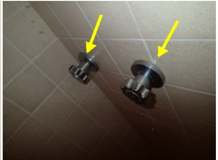
Needs to be sealed.
