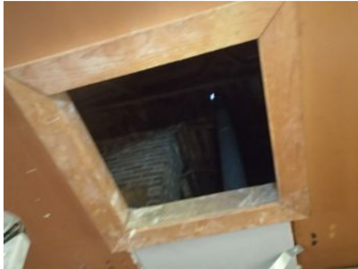
Attic access needs a cover installed.
