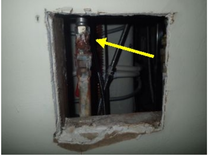
The plumbing for the spa tub is corroded, and starting to leak. I recommend a licensed plumber replace the corroded lines before they fully start leaking.
