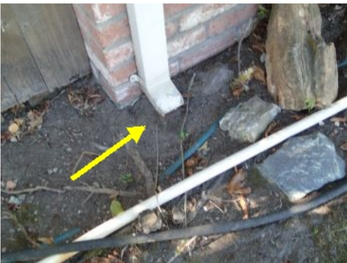
Extensions / Splash blocks missing or insufficient: Install to divert water away from the foundation.
