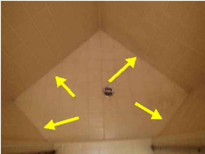
Caulking needed around the perimeter.
