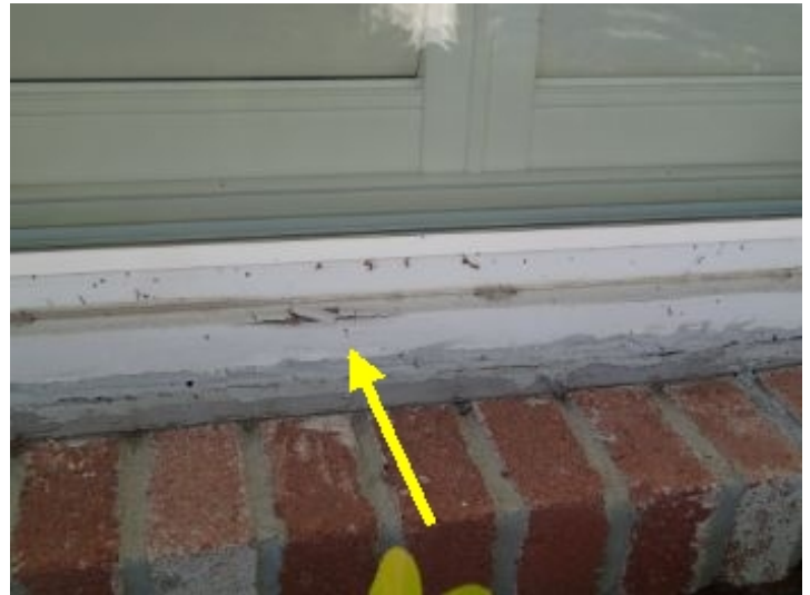
Suggest sealing/caulking as part of routine maintenance to prevent further deterioration.
