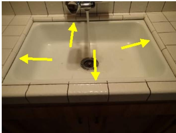
Suggest caulking as necessary.
