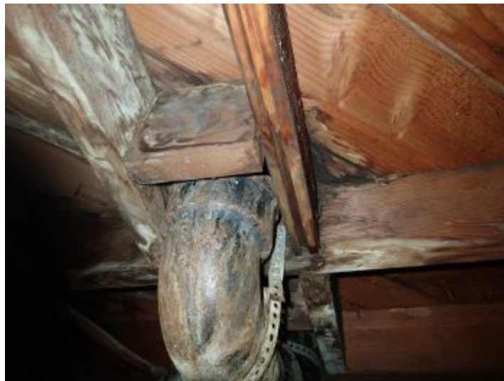
Stains noted under the hall bath.
