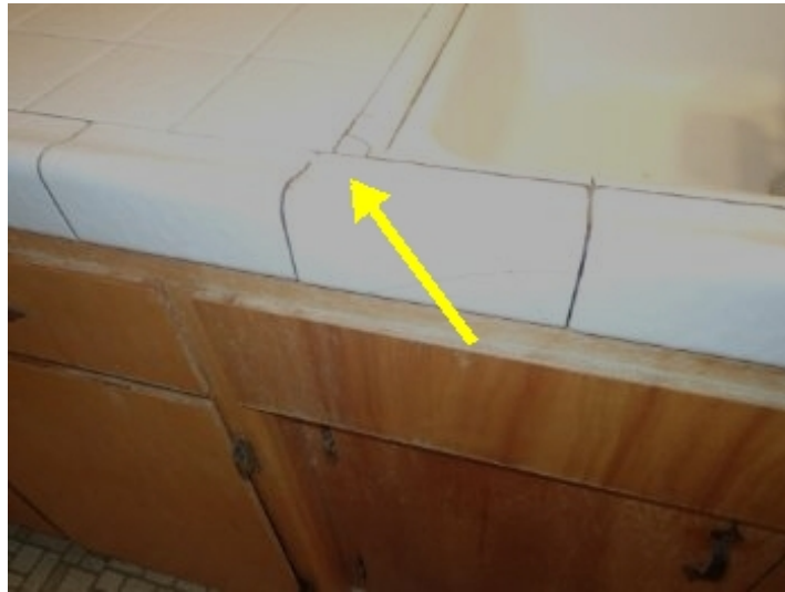
Cracked tiles noted.
