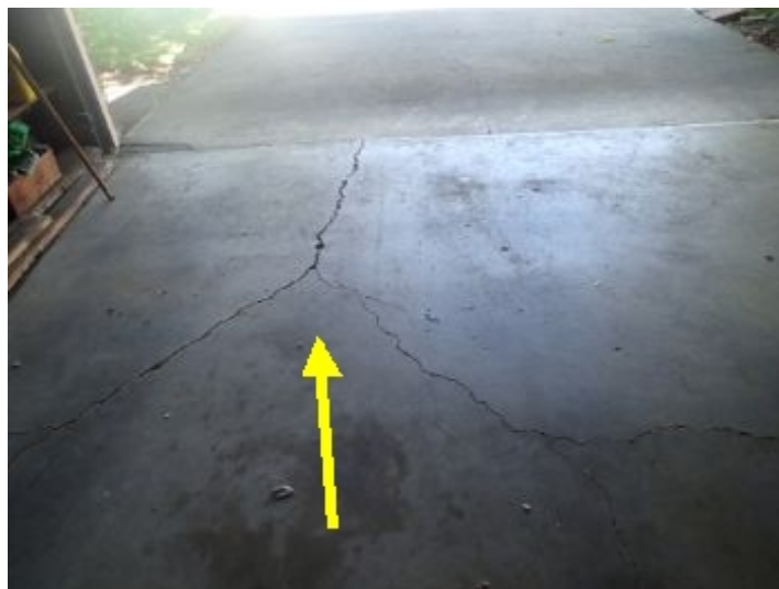
Common cracks noted.
