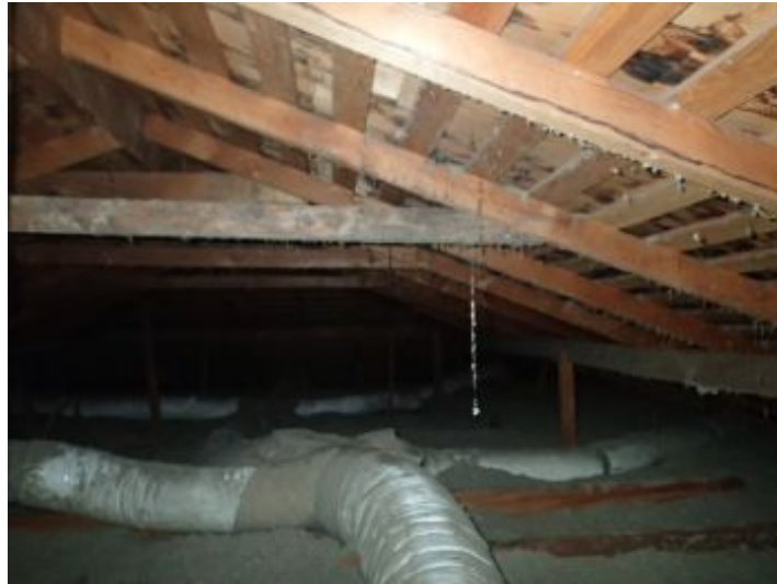
Ducts appear to be in good shape at the time of inspection.
