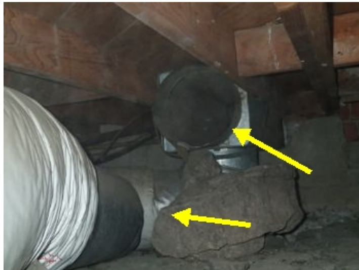
Return air duct is not properly connected to return plenum. I recommend an HVAC company repair.
