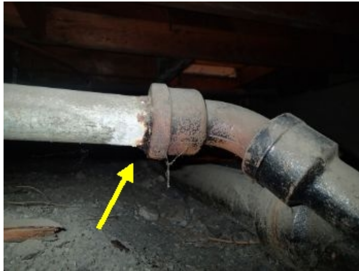
Corrosion/cysts were noted as one or more locations of the metal drain lines. Repairs recommended to be performed by a Qualified Plumber.
