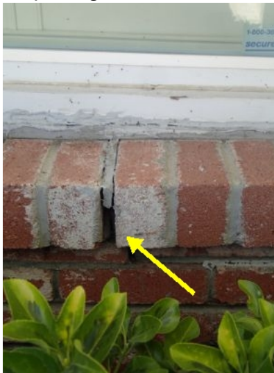
Mortar missing in areas. Recommend repair.
