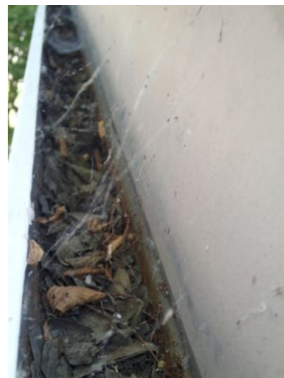
Clean gutters: Significant amounts of debris evident.
