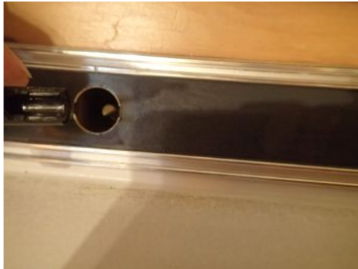
Exhaust fan is inoperable. Needs to be replaced.
