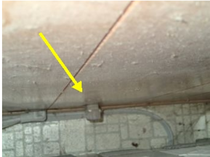
Possible capped gas line behind the stove.
