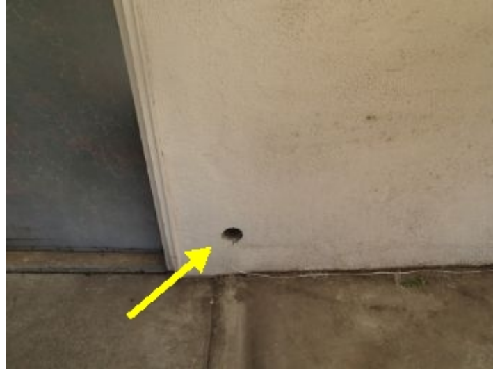
The dryer vent is missing the exterior cover.
