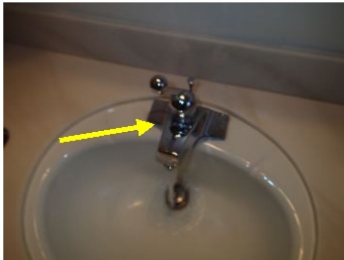
Faucet leaks. Main bath. Recommend replacing.
