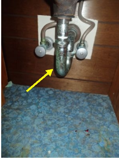
Sink drain is corroded main bathroom. Recommend replacing.
