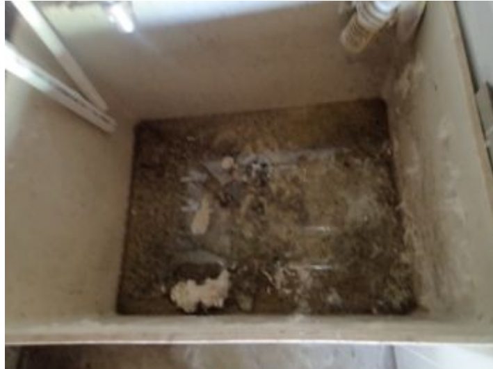
Needs to be cleaned.
