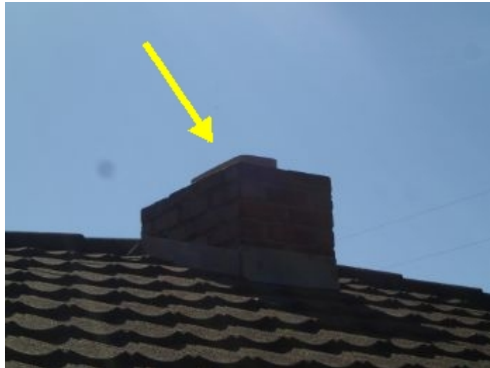
Spark arrestor and rain cap suggested. Main fireplace.
