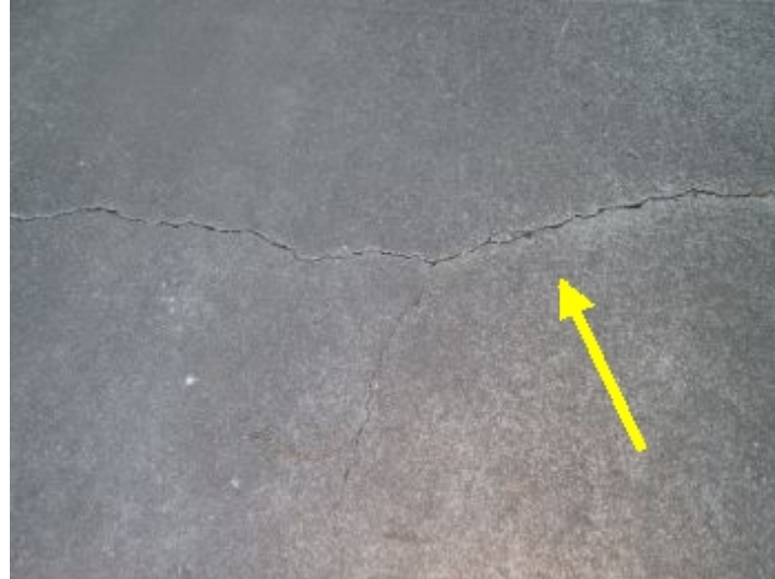
Driveway in good shape for age and wear. Common cracks noted.
